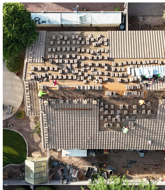
Aerial view of a Tempe tile re-felt in progress. The valleys, perimeter flashing, and tile course alignment are all visible from above. Most homeowners can spot half of these issues from the ground with a phone camera.
